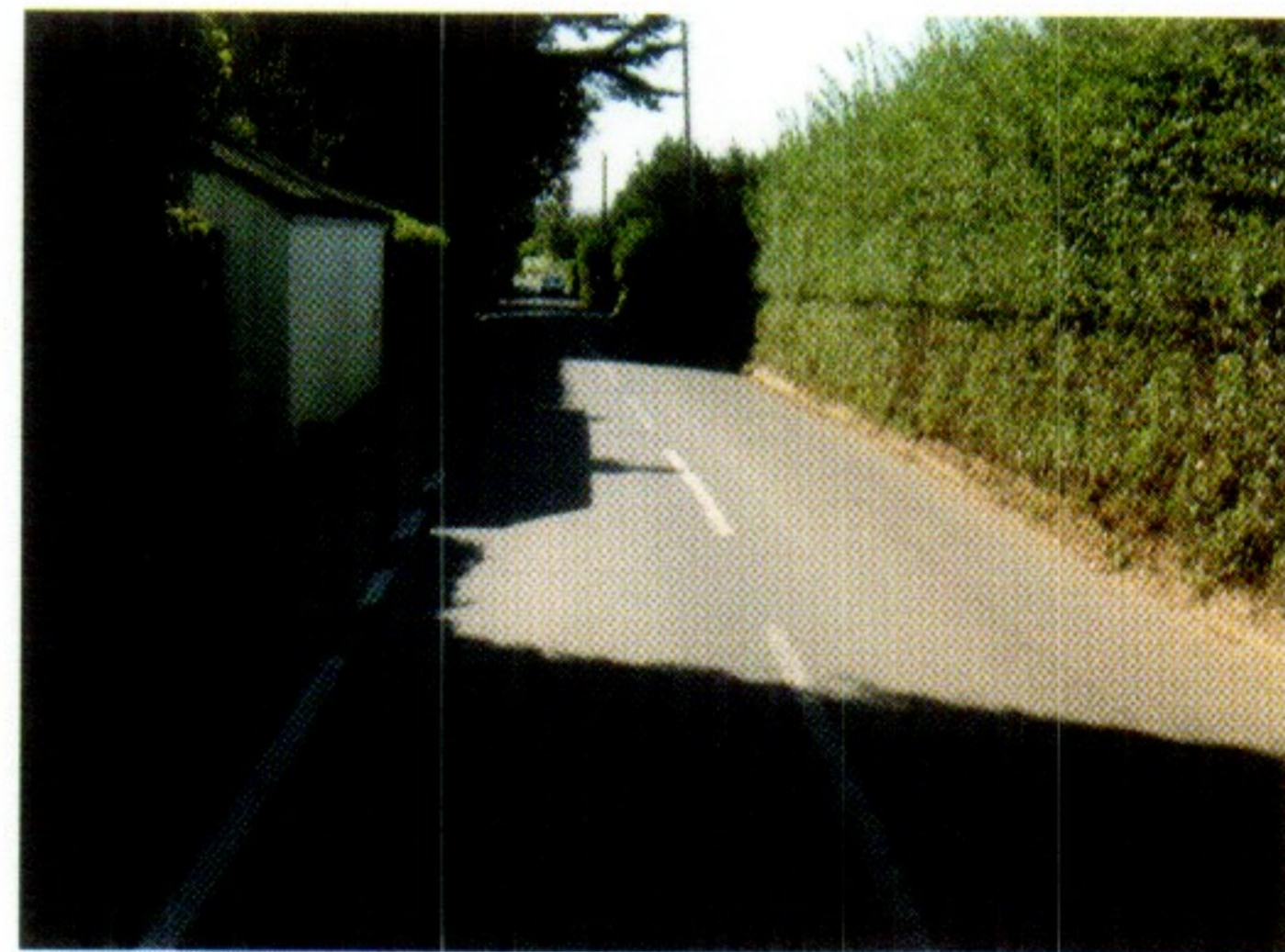
Merstone's lack of footpath/pavement
