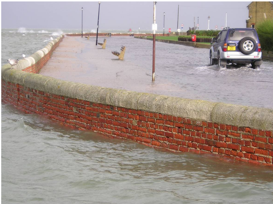
Plate 4: Breach of sea wall at East Cowes (source: Isle of Wight Council)
